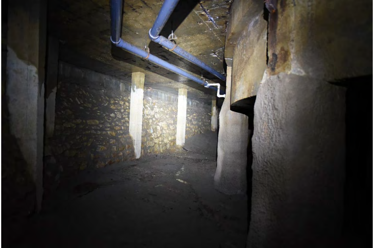
Figure 6. Looking west from the south corner. Stone masonry retaining wall on the left and ahead; pool structure on the right.
