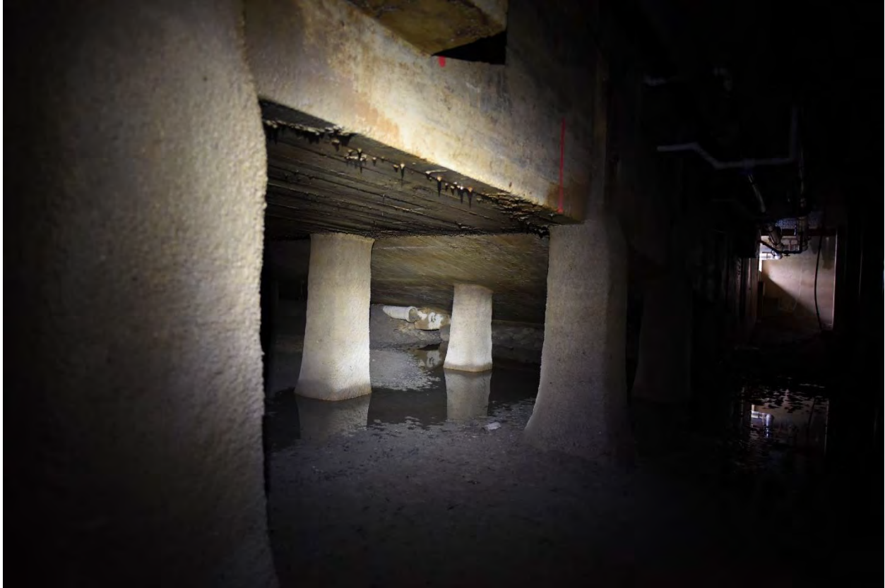
Figure 9. Looking from the southeast side near mid-pool toward the deep end. An unknown PVC pipe is visible in the distance.
