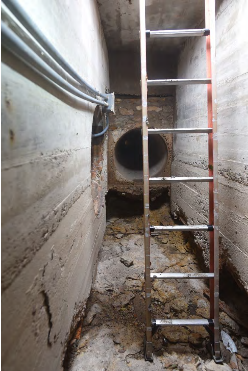
Figure 10. Inside the box culvert on the west side, looking south. The pipe ahead connects to the main spring (Big Chief spring). The opening to the pool basin is on the left. A fissure in the rock is near the bottom of the ladder. Below the pipe ahead, soil is washed out below the pipe and to the left of this is an area of collapsed stone masonry wall (not visible).
