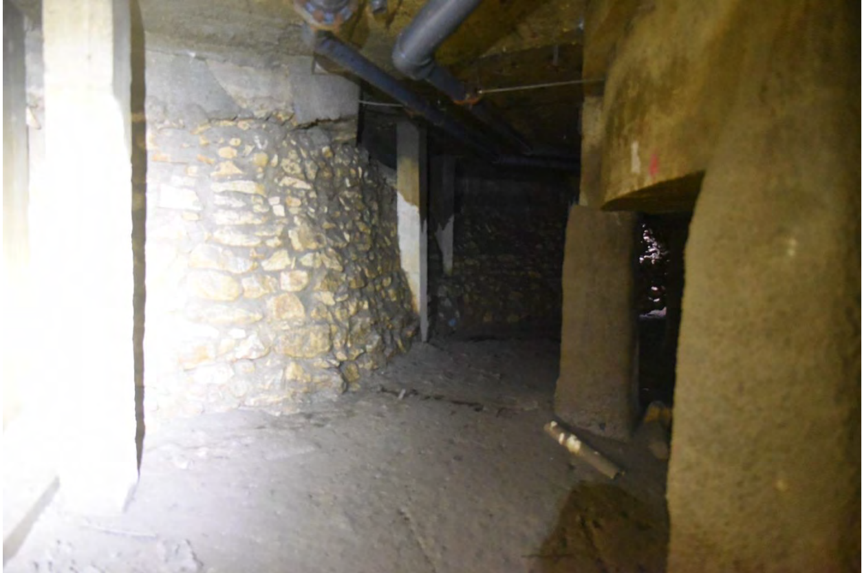
Figure 5. Under the pool deck, looking south toward the south corner. Concrete retaining wall on the left; stone masonry retaining wall ahead, center; pool structure on the right.
