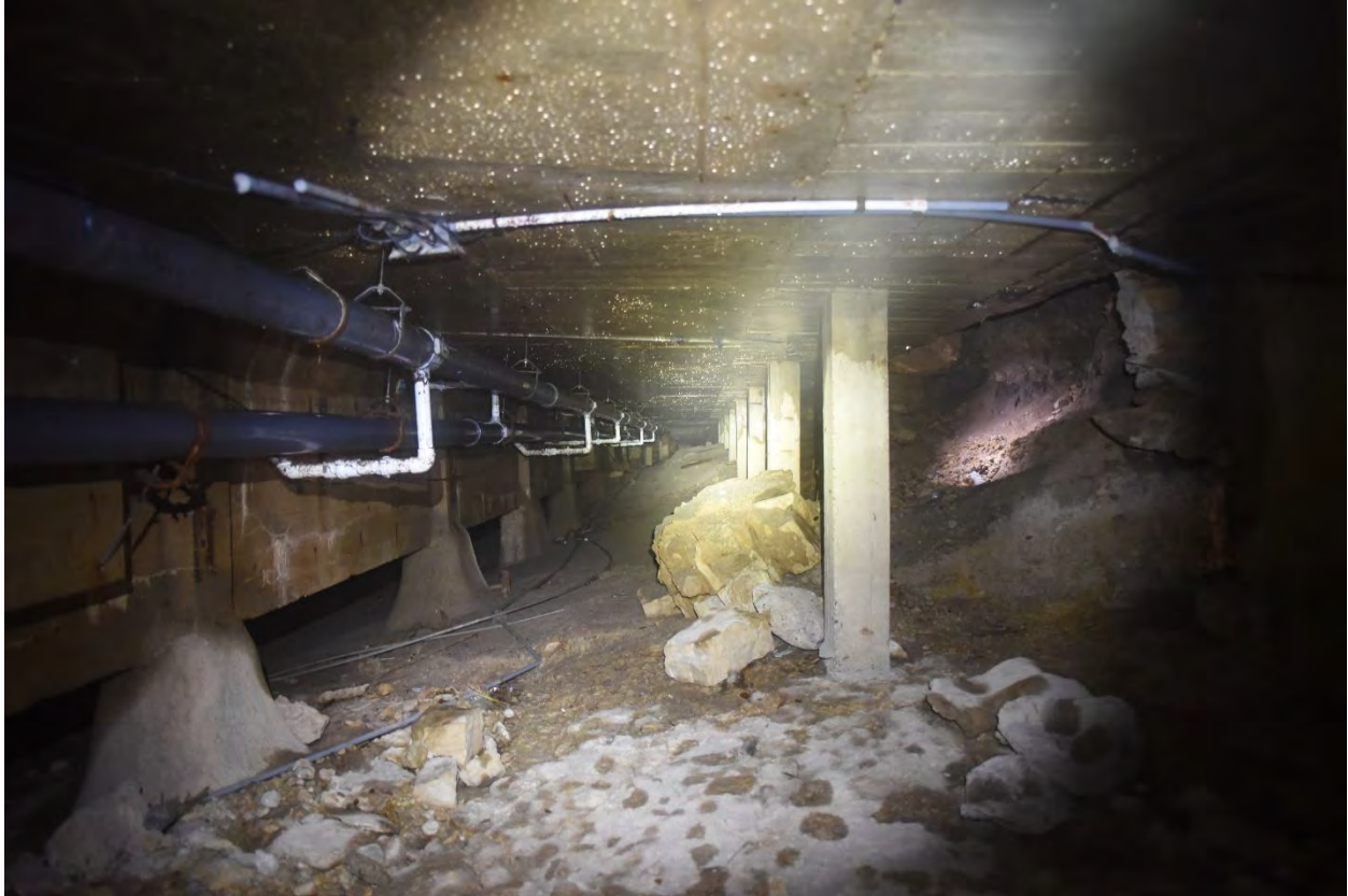
Figure 11. Below the west/northwest side pool deck, looking southwest from the entry point at the box culvert. The pool structure is on the left; rubble of the collapsed stone masonry wall is visible ahead; The retaining wall at the edge of the basin is on the right.
