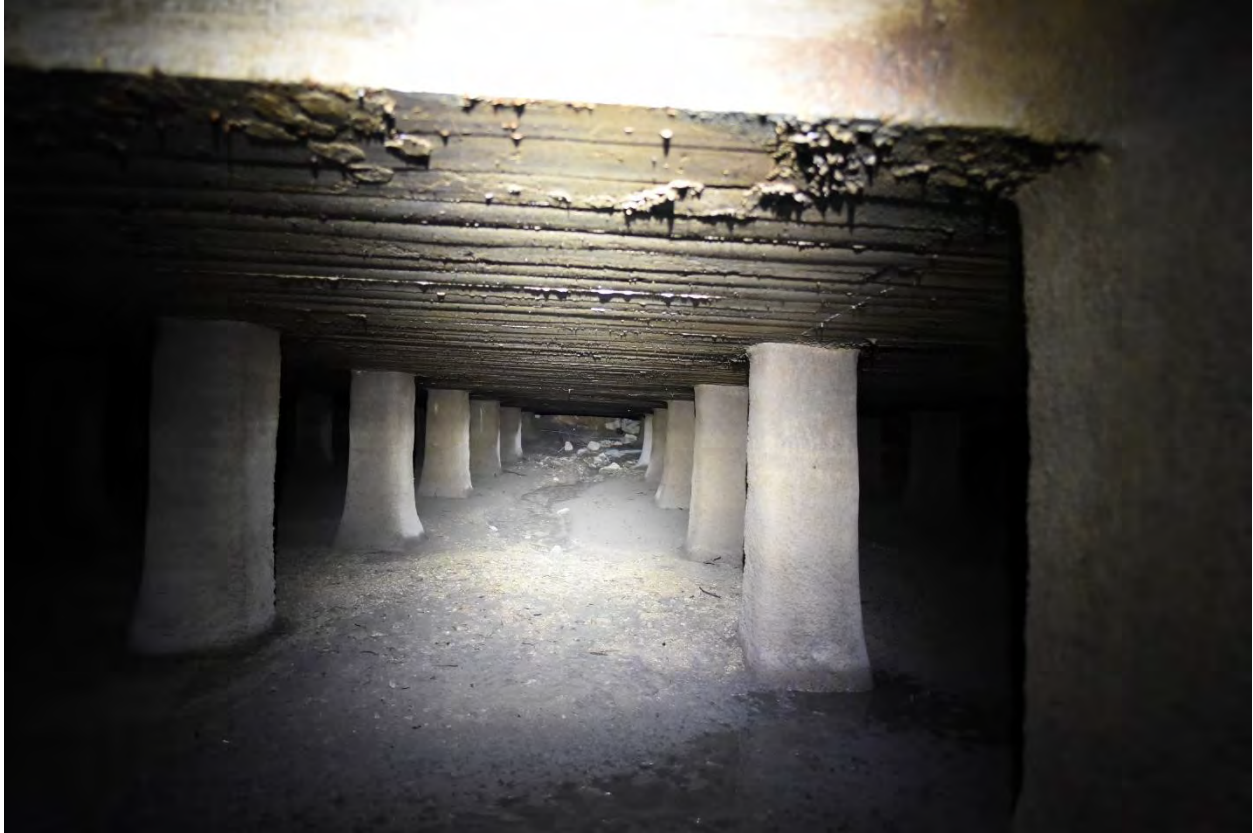
Figure 8. Looking northwest under the pool. The concrete and riprap at the outfall of the box culvert on the west side are visible in the distance.
