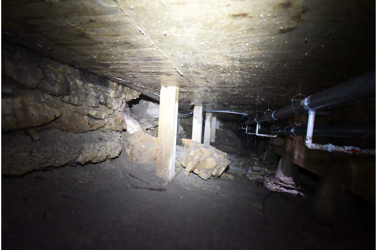
Figure 12. Same collapsed wall segment as in previous figure, looking opposite direction (northeast). Intact stone masonry wall is on the left with the undermined base visible.
