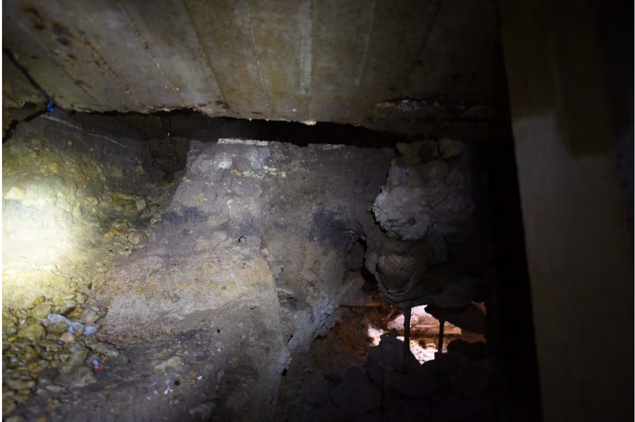
Figure 14. Retained area on west side of basin. The location of the collapsed wall is on the left. The open fissure into the concrete box is on the lower right.
