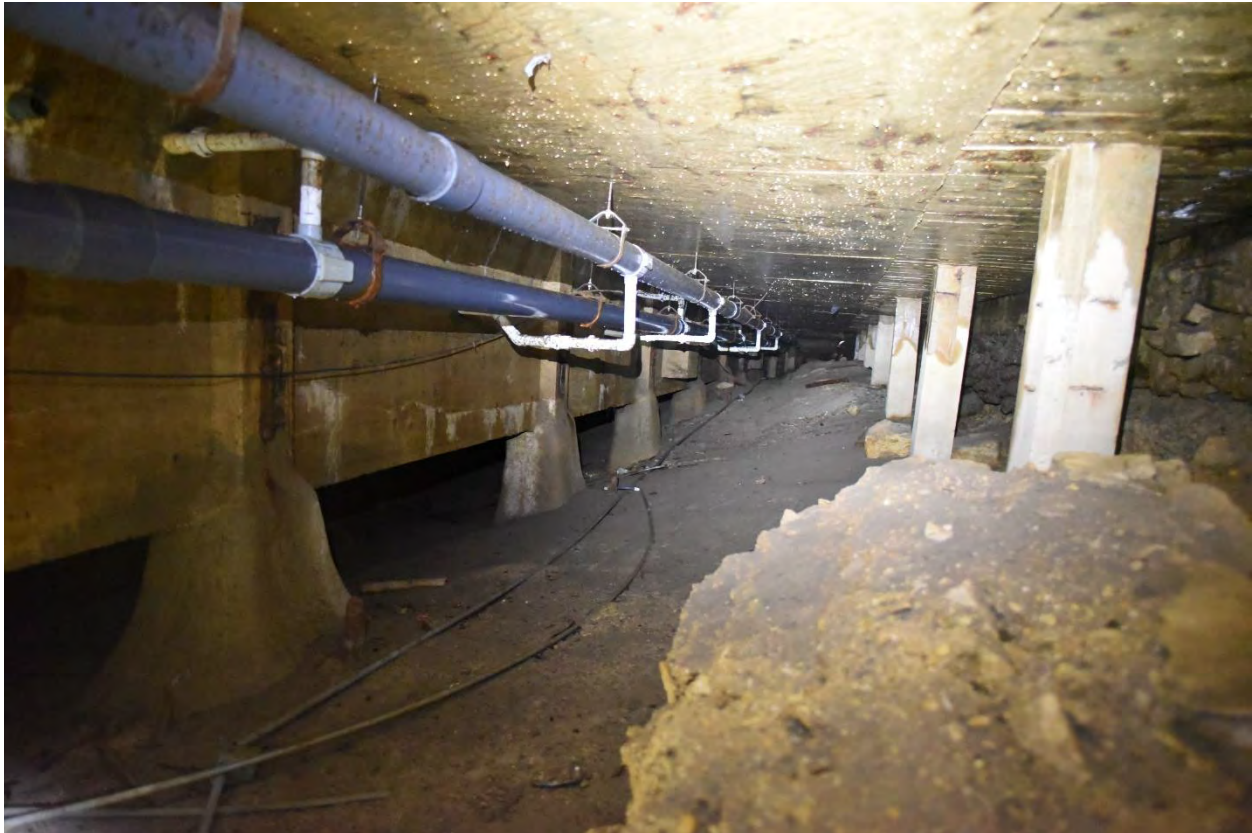
Figure 16. Looking southeast toward the Big Chief spring. Pool structure is on the left; collapsed stone masonry wall in the foreground; retained west side of the basin is on the right. Ahead in the distance, a large diameter concrete pipe is visible to the left of the columns; Big Chief spring is to the right of this.
