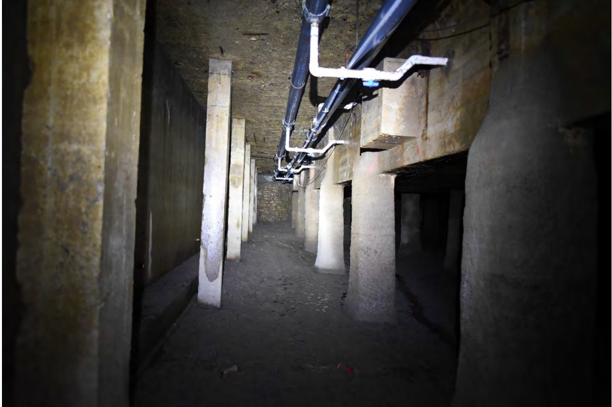
Figure 4. Looking down the southeast side of the pool, from the east corner toward the south corner. Concrete retaining wall on the left; pool structure on the right.
